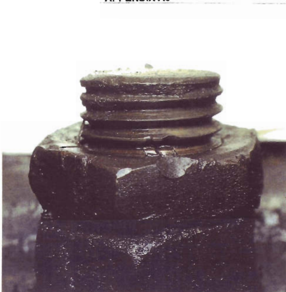
Fig 15 The end of the split pin and damage to the thread on the front right hand M24 bolt of the rear fuel tank
